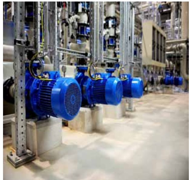
LSB pompen - DWP project, Botlek Nederland
